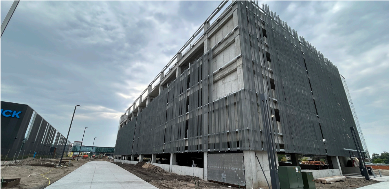
The parking ramp developed in conjunction with the Port Authority and SICK.
