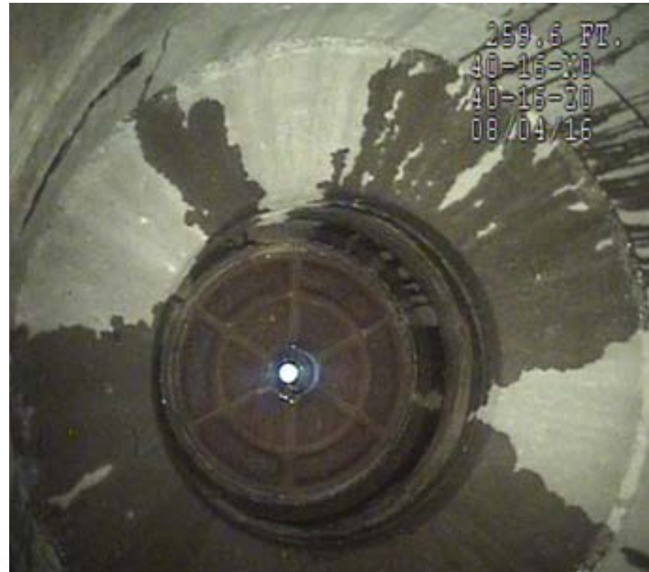
Example of an Unsealed MH During a Rain Event
