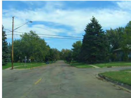
As this photo illustrates, a 2-lane configuration is found on the eastern end of West 110th Street.
